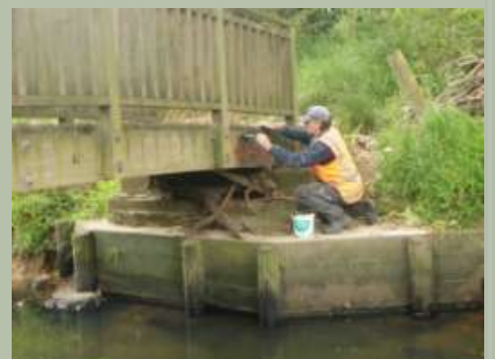
Graffiti busting at the bridge.
