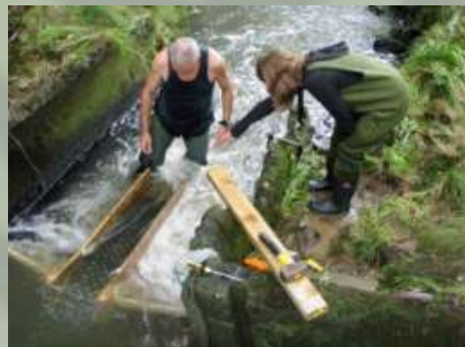
Pete Pattinson and Catriona Paterson installing the fish ladder at the Water Flow Monitoring Weir.
